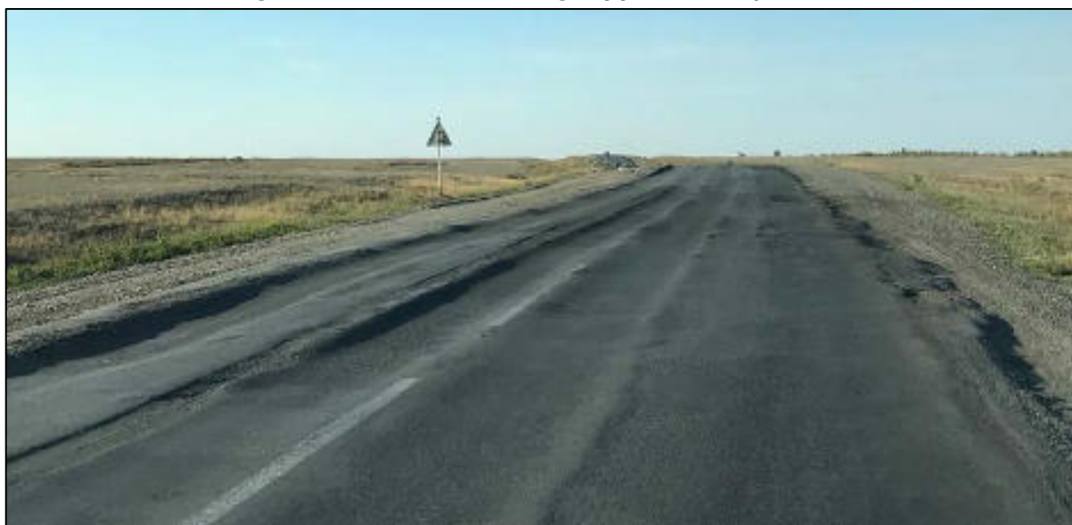
Figure 5: Pavement Rutting, Approximately KM 80
