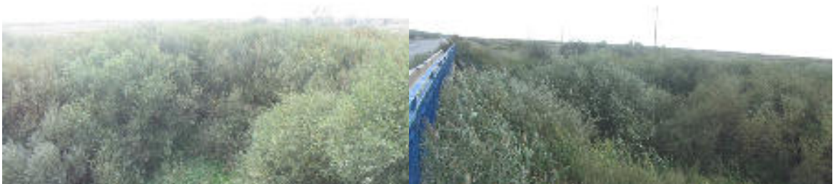
KM67. Bridge over Talasbay river – riverbed is dry from both sides of the bridge and densely vegetated mainly by willow, oleaster, reed, gooseberry bushes
