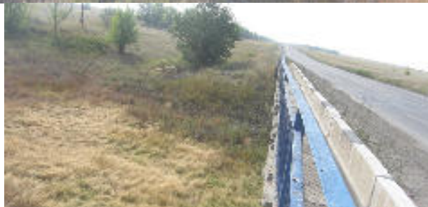
Plate B.7: KM24+98 - The following bridge structure is in the form of a reinforced concrete two span beam bridge across the dry bed of the tributary to the Aktobe reservoir. The bridge has a rectangular shape and is oriented from the north-west to the south-east. The length of the bridge is 37.40 m, width - 8.15 m, width of the carriageway - 8.3 m, height - 4.3 m.
