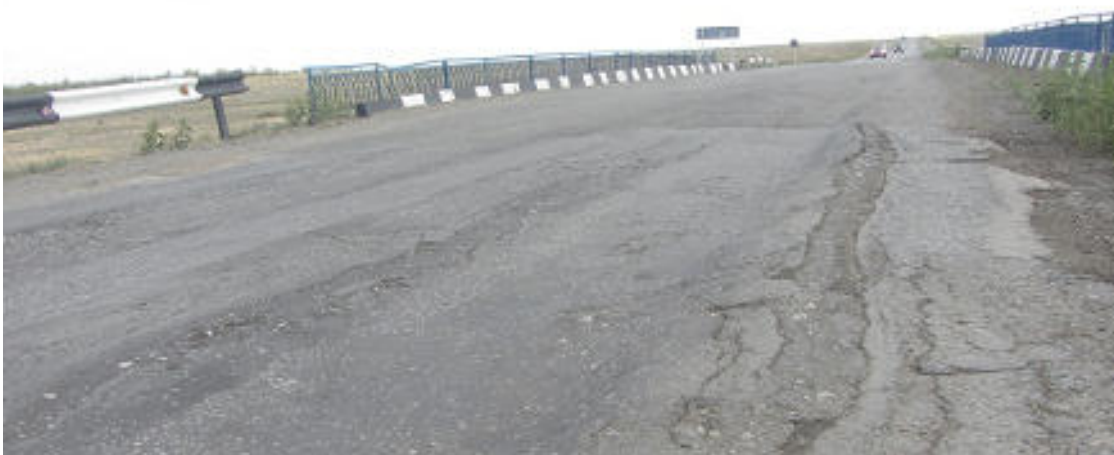
Road surface is heavily deteriorated
