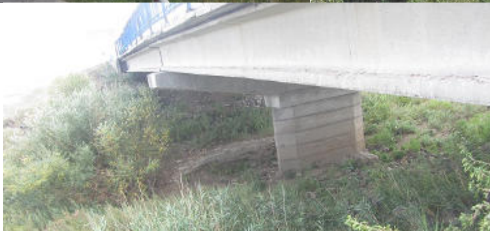
KM79. Bridge over Tabantal river – riverbed is dry currently from both sides
