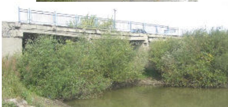
Plate B.11: KM35+50. The road crosses Batpakty river via three span beam reinforced concrete bridge. The bridge is oriented from the north-east to the south-west, has a rectangular shape (8.15 × 21,0 m), height is 3.7 m. The bridge has asphalt concrete covering, the width of the carriageway is 5.30 m, pavement part has a width up 1.0 m. Condition of asphalt concrete pavement and pavement part of the bridge is unsatisfactory, there are deformations and fractures can be observed. There is a metal rails with a height of 1.2 m from both sides of the bridge. River bed is almost dry (only
