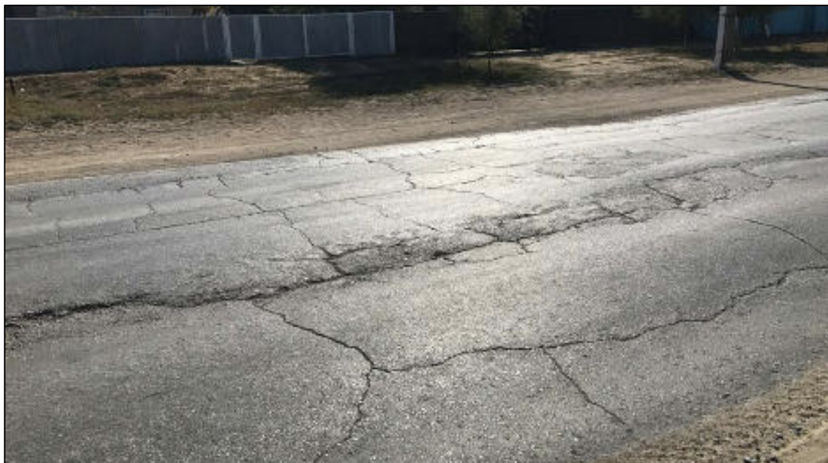
Figure 6: Cracked Pavement, Bestamak
